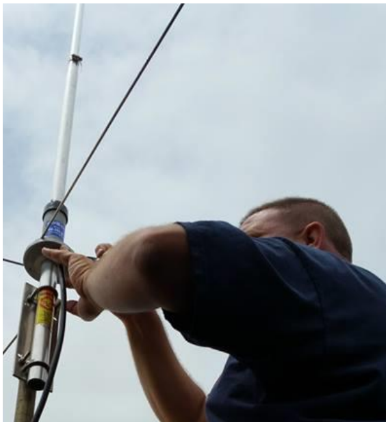
Who is this masked antenna installer? Why, it's Tom KB2GTO, installing our Repeater's new antenna!
